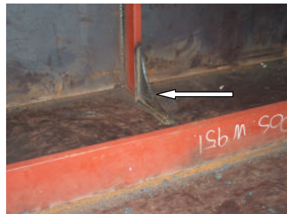
Figure 5, DMA went through all details as they usually do when inspecting ships. A bulkhead stiffener had to be changed in order to have more smooth stresses. Furthermore, additional requirements regarding implementation of safety instructions were given.
